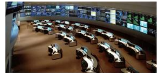
The Network Operations Center (NOC)
